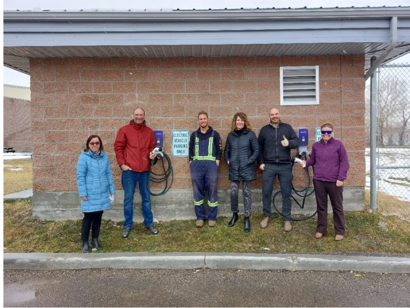
Figure 3: Recreation team standing with EV chargers installed with the support of Enel Green Power and Southgrow
