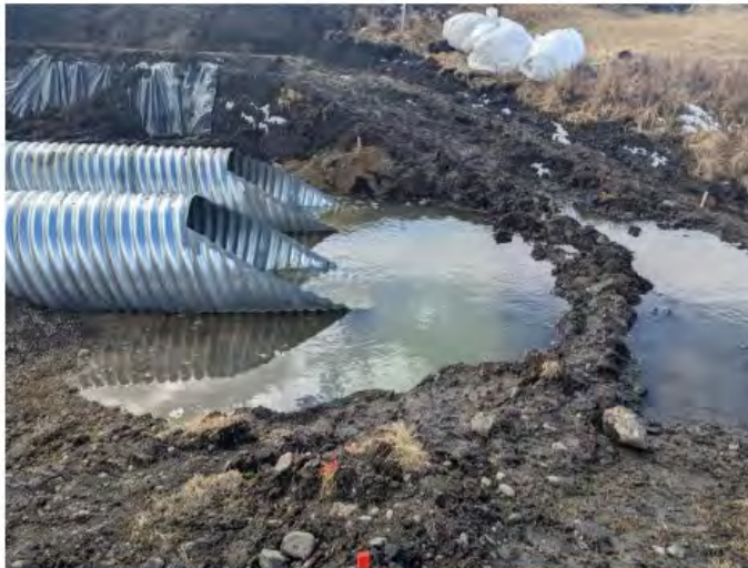
April 3, 2026 Post Isolation Breach, down stream end.
