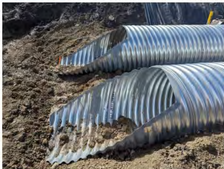
April 3, 2026 Post isolation breach upstream end
