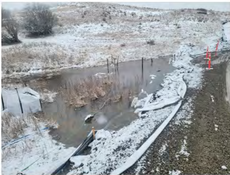
April 2, 2026 Isolation Breach.
